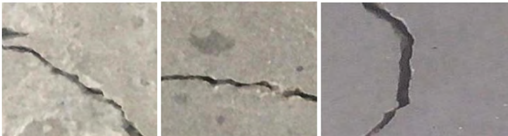
Fig. (1). Surface images with crack.
