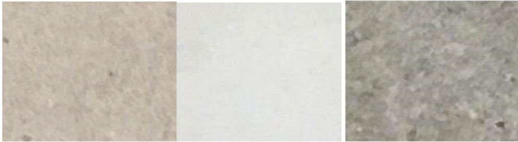
Fig. (2). Surface images without crack.
