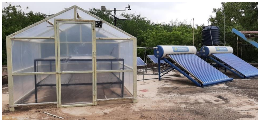
Fig. (2). Actual view of installed PVT-hybrid greenhouse dryer.
